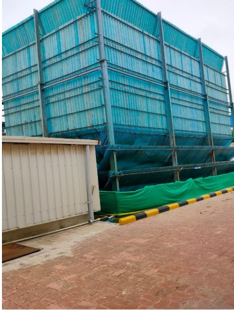
MIST COOLING TOWER
