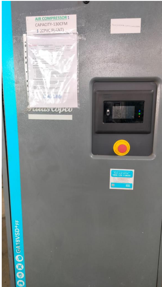
VFD OPERATED COMPRESSOR SYSTEM
